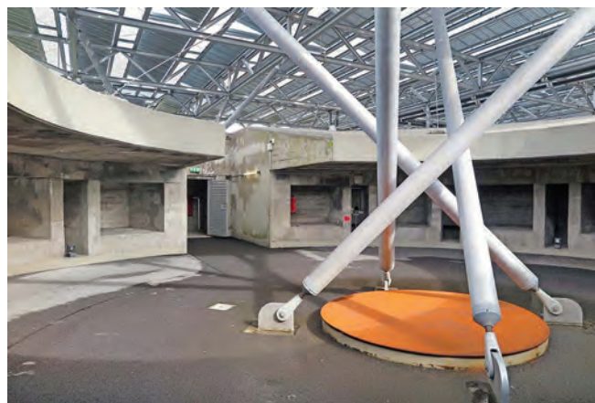
On the roof of Wilhelmsburg Flak Tower in one of the original gun emplacements. The modern struts support a solar panel array.
